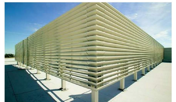
5. PENTHOUSE EQUIPMENT - SCREEN
