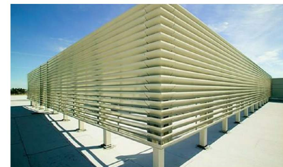
5. PENTHOUSE EQUIPMENT - SCREEN
